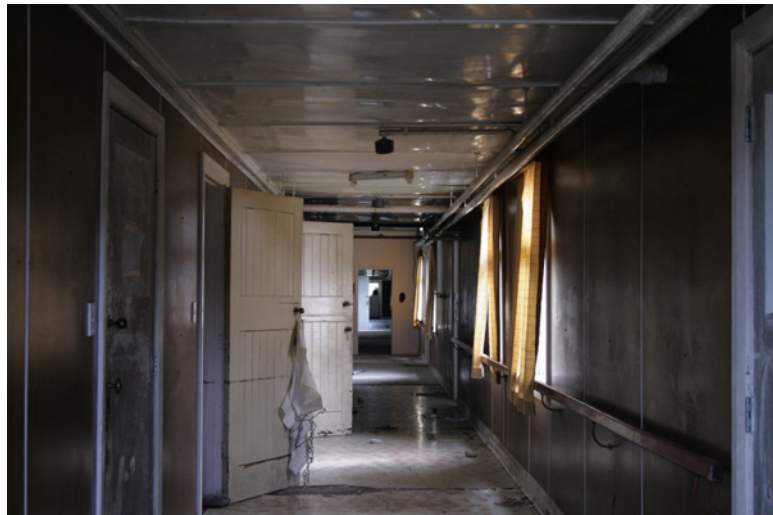
Figure 1 The corridor of a patient villa at Seaview Asylum, Hokitika, New Zealand. Photograph by author, April 2010.
