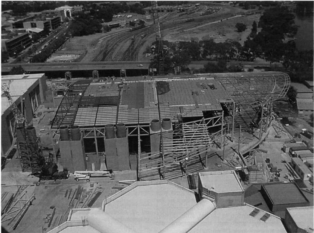
Figure 1: Progress of the ACC EXT-over the track of the railway Courtesy of Mr. Paul Schlosser; Baulderstone and Hornibrook
