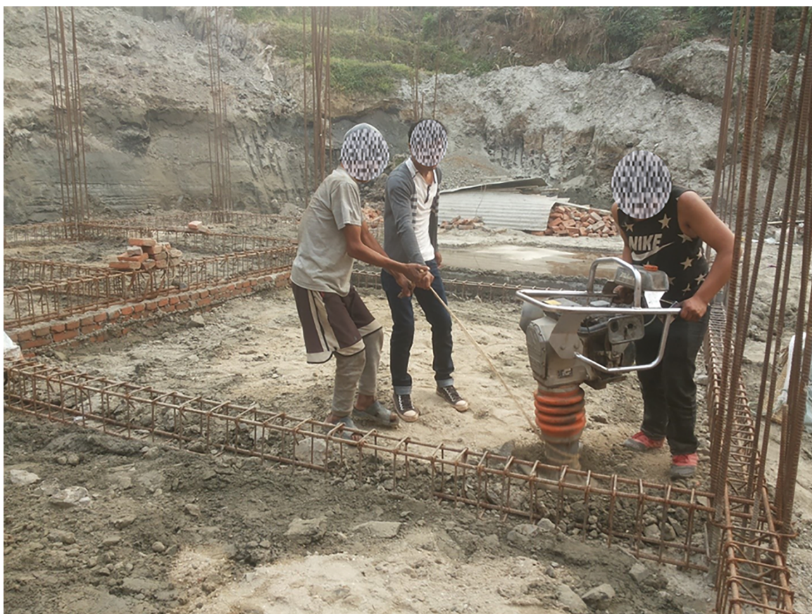
Figure 2. Workers with no Safety Equipment in an Active PDR Site in Bhaktapur, Nepal
