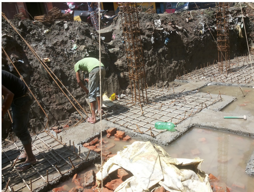
Figure 3. Unmanaged Debris and Wastes on an active PDR Site in Bhaktapur, Nepal
